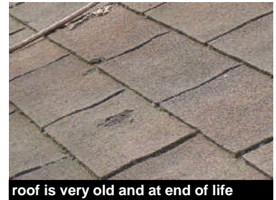
roof is very old and at end of life
