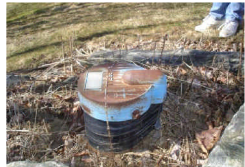
temporary well cap - health concern
