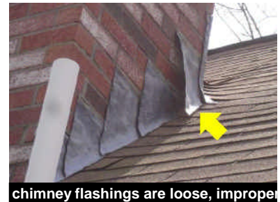
chimney flashings are loose, improper
