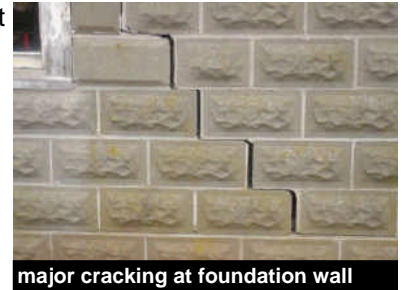
major cracking at foundation wall
