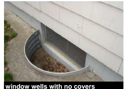
window wells with no covers
