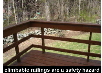
climbable railings are a safety hazard
